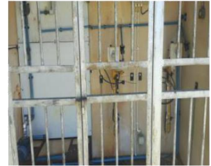
Chlorination system not functional, there is no chlorine.
