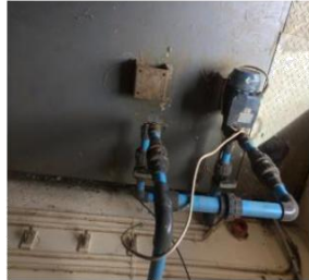
Water booster pump not operating
