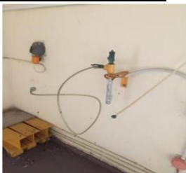
Chlorine room, gas controller is missing
