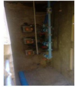
Two pumps missing, housing assemblies and liners are not working.
