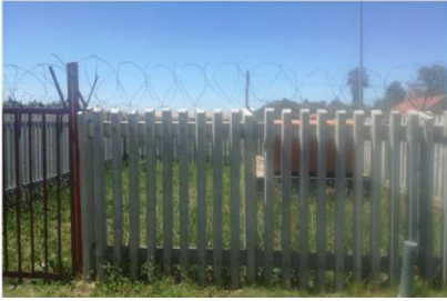
Overview of the pump station
