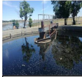
Secondary settling tank not functional
