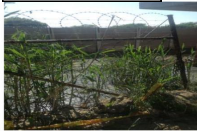
Lots of flooding, pump station not working
