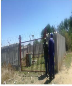
Argon Pump station
