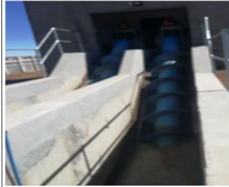
Screw pumps, fully operational
