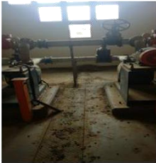
No electricity at the digesters pump station
