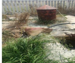
Submersible pump being used for now.
