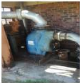
Pump 1 fully operational
