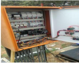
Panel Box fully operational
