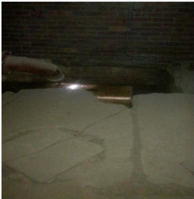
No pumps and DBS.
