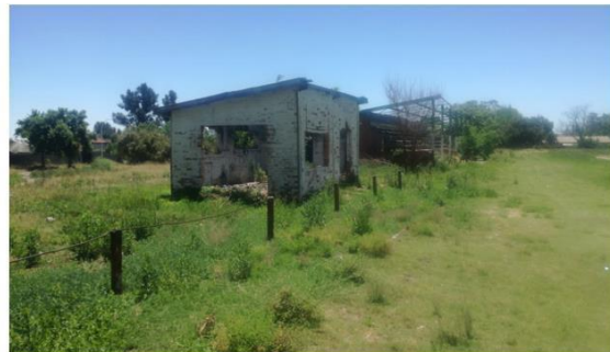
No proper fencing around the vandalised building
