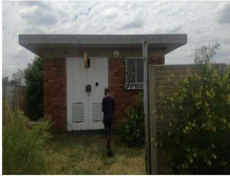
The pump station does not have a gate
