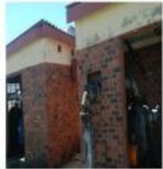
Buildings in poor condition.
