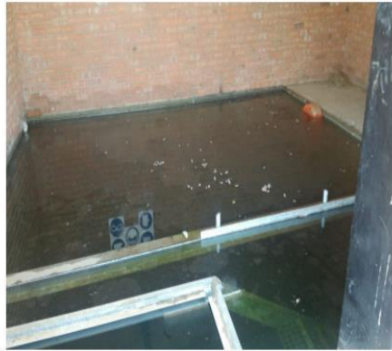
Inside it is full of water and no pumps
