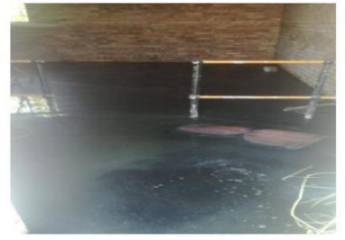
Flooding inside the pump station
