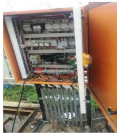
Panel Box fully operational
