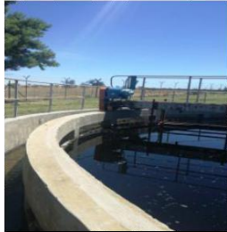
Burnt motor at secondary settling tank
