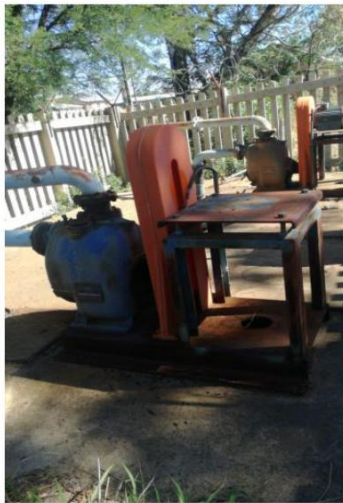
One pump does not have motor
