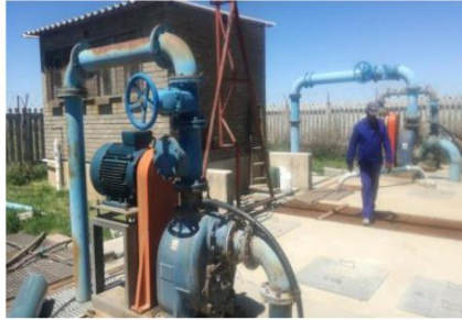
No power supply, no clean water and no sewer
