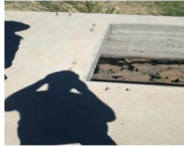
Stolen rails chlorine tank
