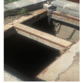
One temporary pump currently being used.
