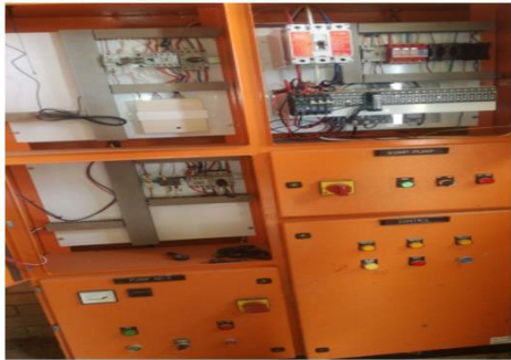
Panel, fully operational
