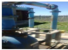
Motor and assembling missing in pump 4
