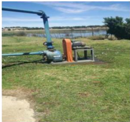
Impeller pump fully operational
