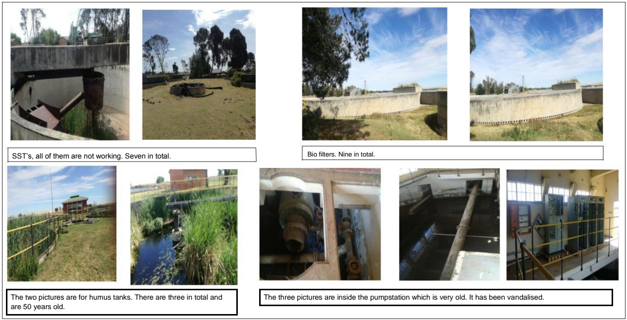
Theronia WWTW (continued)
