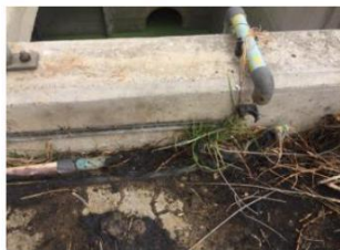
Pipe supplying chlorine burnt by vandalism
