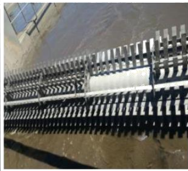
Brush aerator, motor not functional
