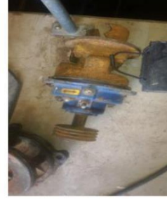
Two assemblies missing in two pumps
