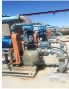
Pump station has not been functional for the past 5 months
