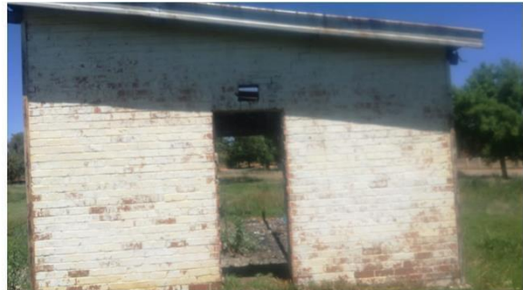
The building need to be demolished and reconstructed.
