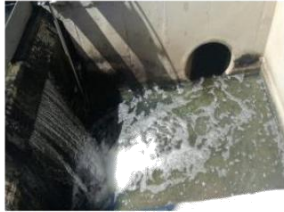
Out flow fully operational
