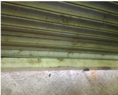
Thieves lift the roller door to gain access into the station
