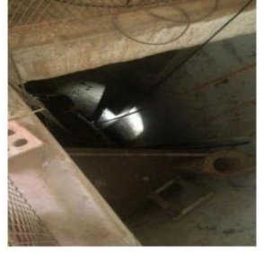
3 pumps, only 1 pump working, the other 2 do not have motors
