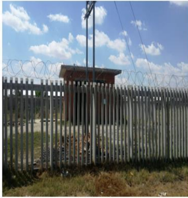
Hani Park Pump station
