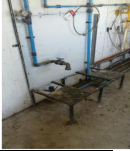
Chlorine tank missing, booster pump stolen, still waiting for the order.
