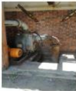
Pump 2 fully operational
