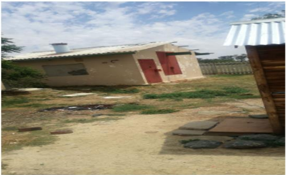
No keys to the gate, there are two pumps but only one working. The other pump does not have motors
