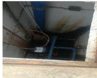
Two pumps only one pump working, the other one does not have a motor
