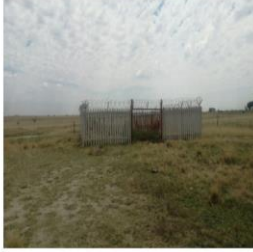
Ben Regal Pump station
