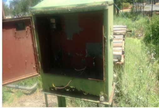
Vandalised switch box for booster pumps
