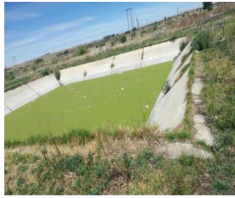
Anaerobic pond not operational
