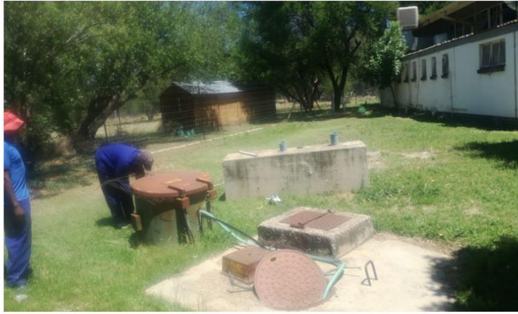
Pump station inside Tikwe lodge ,one pump functional.
