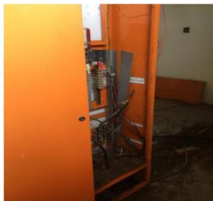
Stripped panel box
