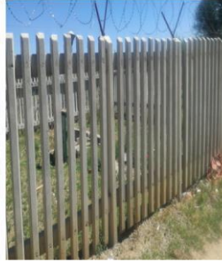
Concrete palisade fencing not safe from vandalisers.
