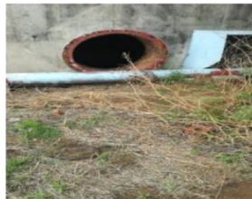
Stolen pipes at digesters
