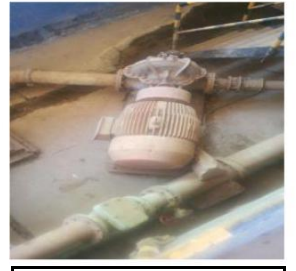
One of the two pumps not working
