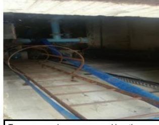
Two pumps only one pump working, the other one does not have a motor
