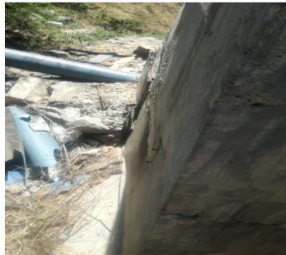
Vandalised not working
