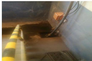
Sump pump, fully operational
