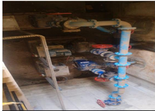
1/3 pump working, the other two pumps are not working, no motors and rotation assemblies
