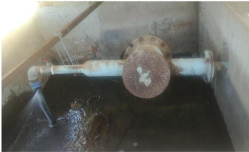
Pump not operating
