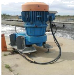
4/6 generators at aerobic tanks not working due to cable theft
