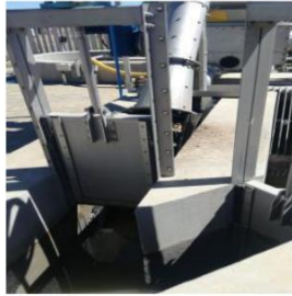
Mechanical screen fully operational
