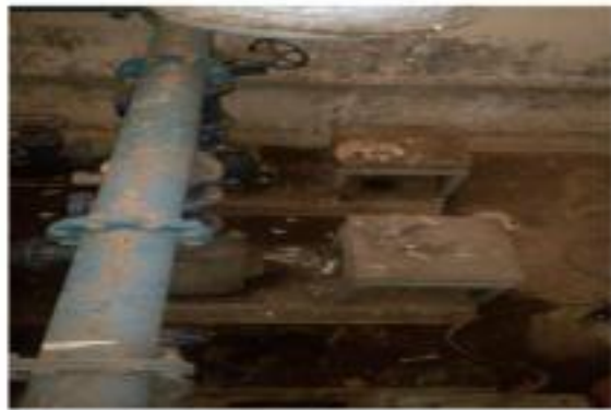
2 pumps not working, no rotation assemblies and motors
