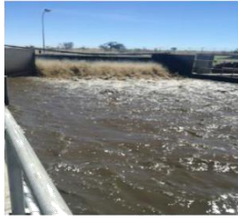
Aeration tank functional
