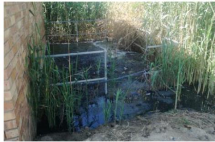
Pump station sumps not working
