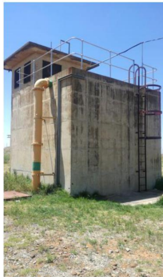
Old hennenman pump station inside yard
