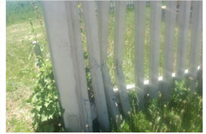
Broken concrete palisade fence
