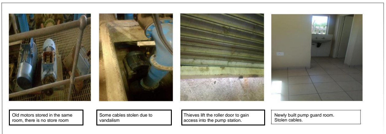
Hoof Pump station (continued)
