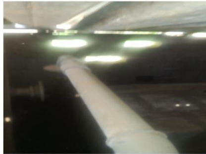
No motors, pump stolen and vandalised
