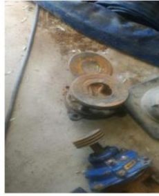
Ware-plates missing in two pumps
