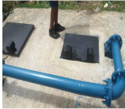
Only submersible pump currently not working
