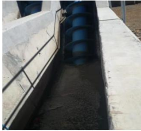
Both screw pumps working well
