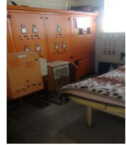
Panel missing, currently using the two panel boxes
