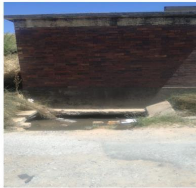
Side view, station vandalised
